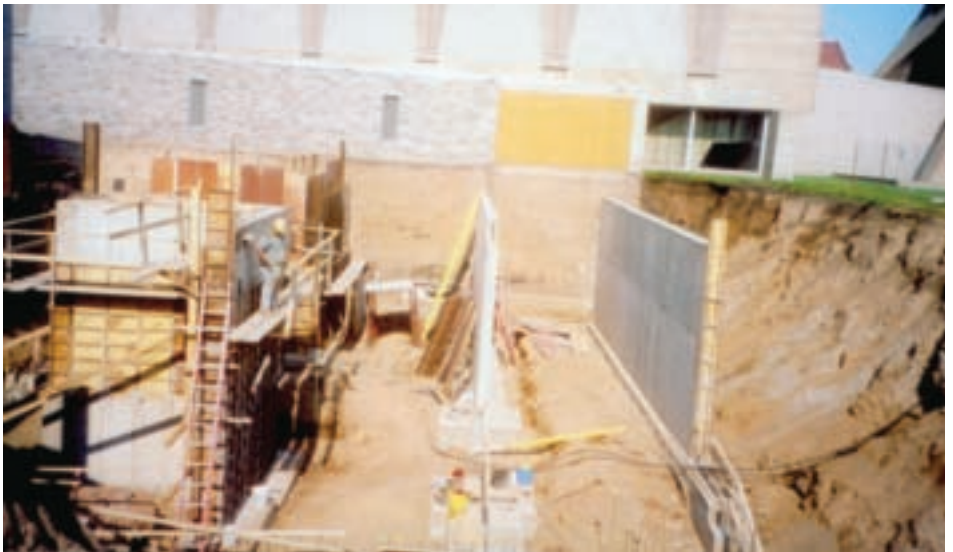
An early July photo of the tunnel link between the Petters Pavilion and the Abbey Guesthouse
